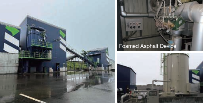
Intermediate Treatment Facility at the Teraji Plant
