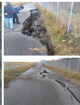
Noto Airport Damage Sustained at Noto Airport
