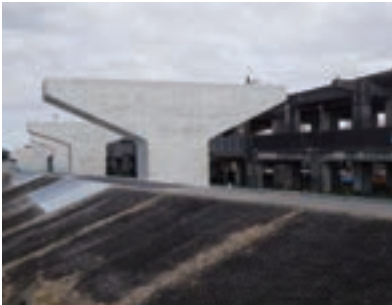
Chiba Prefecture Comprehensive Social Capital Grant Construction (Tentative name: Tsuchiyabashi Main Line P10, P11 Bridge Footing) (Chiba Prefecture)
