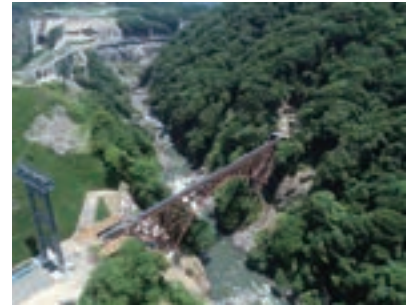
MM BRIDGE CO., LTD. Dai-ichi Shirakawa Bridge Restoration Project (Part 2-1) (Kumamoto Prefecture)
