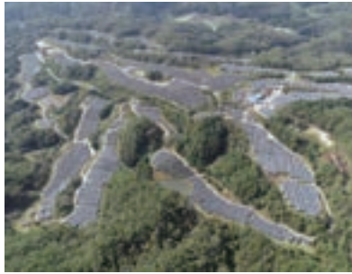
Hitachi, Ltd. SGET Hiroshima Mega Solar Power Plant Construction Project (Hiroshima Prefecture)
