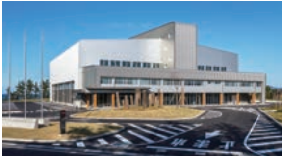
Joetsu City Tentative name: Joetsu City Gymnastics Arena Construction Project (Niigata Prefecture)
